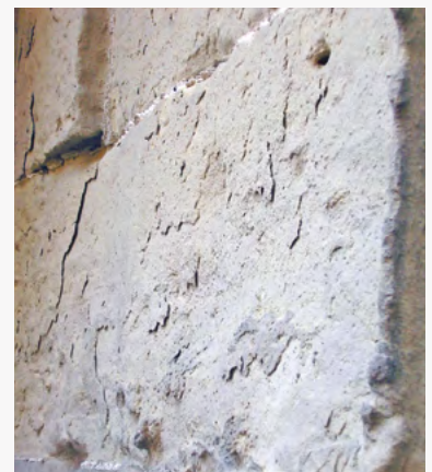
Some examples of degradation of exposed walls.
